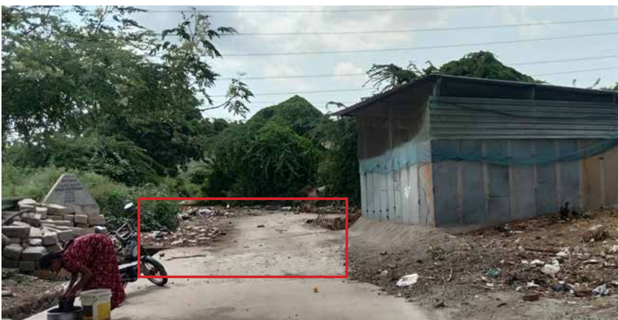
Stretch of road extended to facilitate drainage and keep the path to the fields clear of water logging
